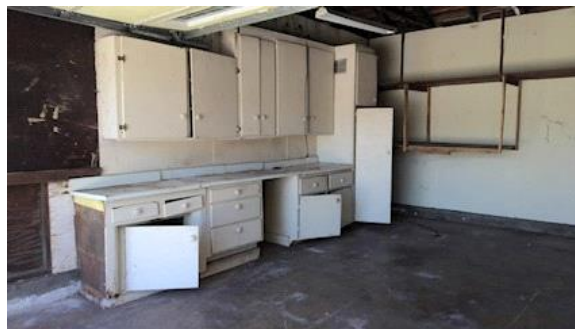
Decayed / damaged built in cabinetry
