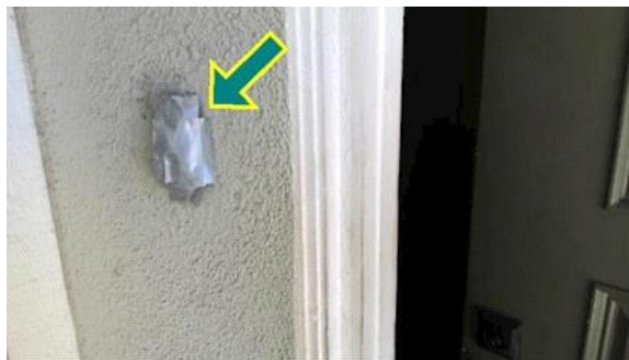
Altered / inoperable (unconfirmed) doorbell
