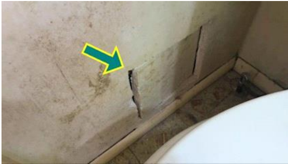
Altered / penetrated wall board
