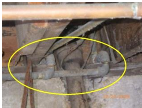
Old galvanized pipe still present
