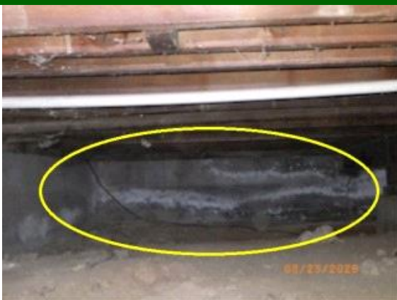
Efflorescence / chalky substance present
