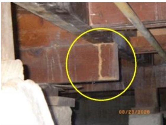
Ex.#2: Wood rot / suspected termite conditions @ framing & support
