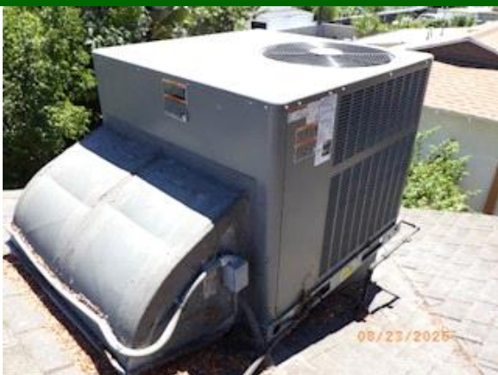
RTU combo system observed intact & functional
