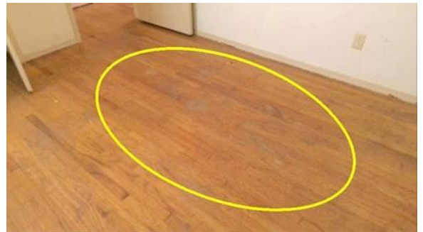
Bedroom 2 / Interior view #2 - Scratched, marred wood flooring
