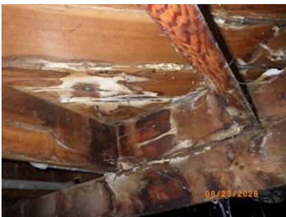
Stained / deteriorated wood conditions
