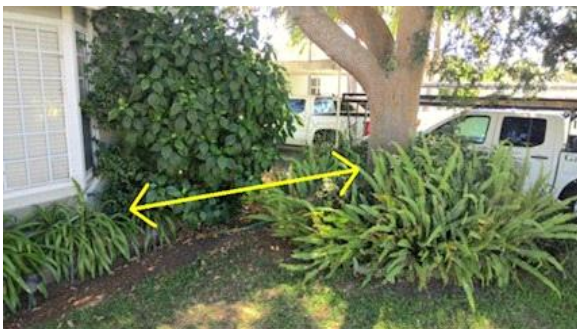
Tree root proximity to foundation
