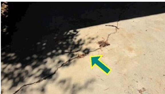
Cracking conditions observed
