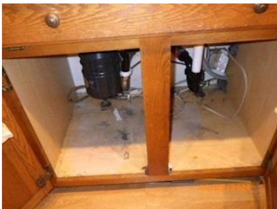
Ex.#1: Stained / deteriorated surfaces below kitchen sink
