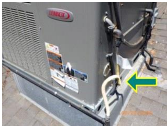
Observed CSST @ RTU
