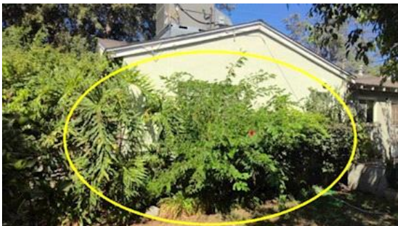
Obstructed access &/or visual of external siding
