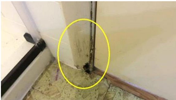
Decayed entry door trim
