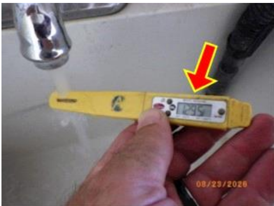
Water temperature exceeds 120 degrees
