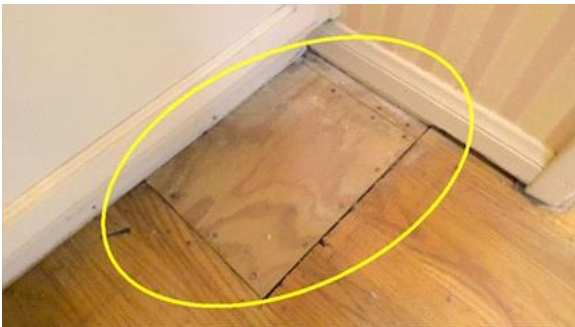
Unfinished flooring patchwork
