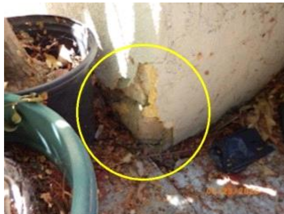
Damaged / penetrated stucco surfaces
