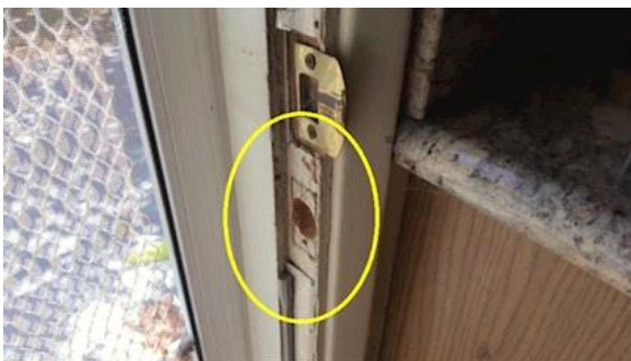
Missing latch plate
