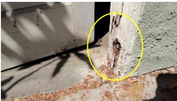
Wood rot, decay and/or suspected termite related conditions
