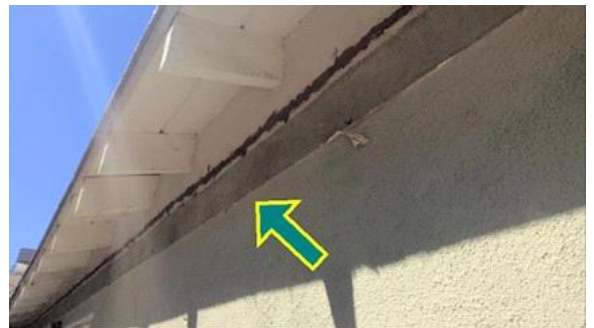
Altered, penetrated & unsealed stucco surface areas
