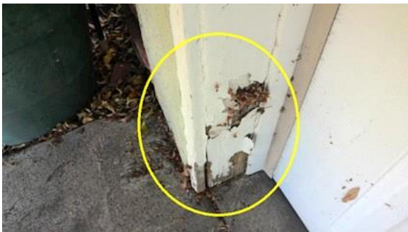
External surfaces in need of servicing, paint and/or sealing
