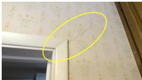
Diagonal cracking above door
