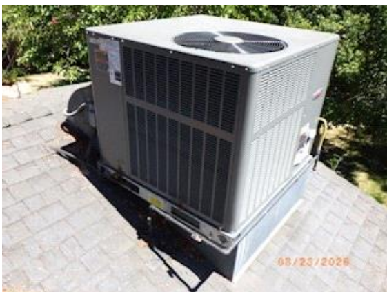
RTU system observed secured & intact
