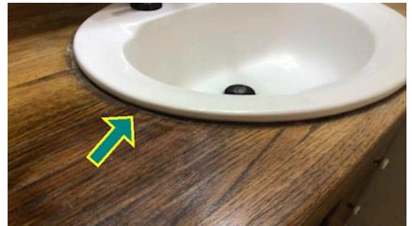
Basin loose & lifting
