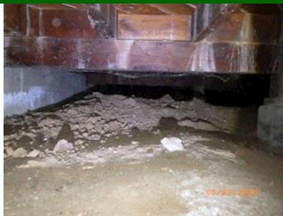
Ex.#2: Limited / obstructed interior access & visual inspection
