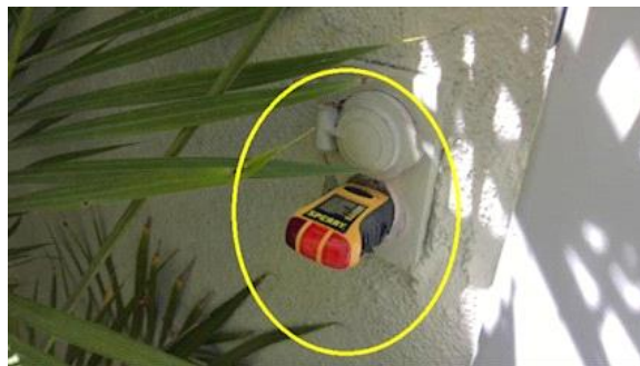
Weatherproof enclosure damaged / Open ground detected
