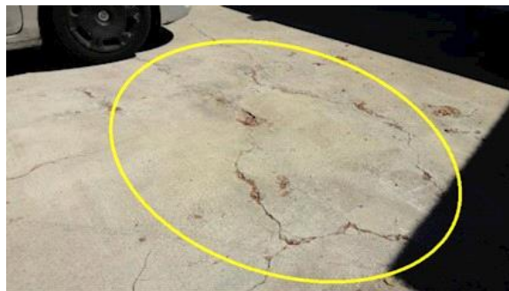
Indented / eroded concrete
