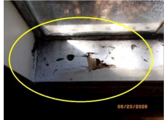
Additional example: Rotted / decayed window sill surfaces @ family room
