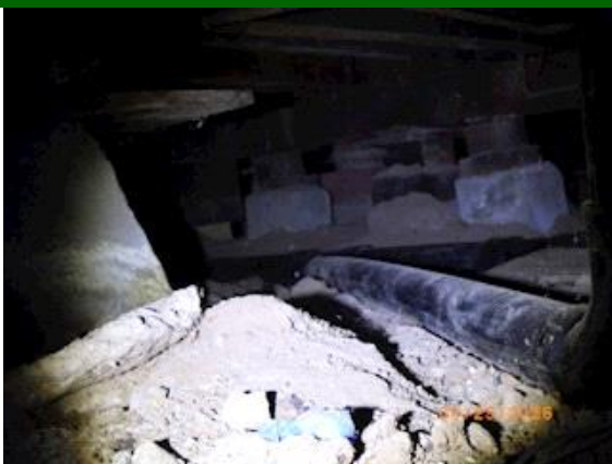
Ex.#1: Limited / obstructed interior access & visual inspection
