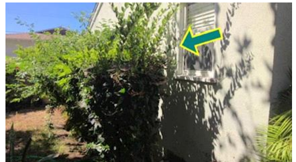
Vegetation in contact with siding
