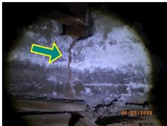
Suspected termite tube & efflorescence / chalky substance present
