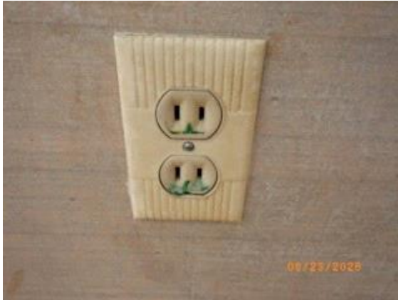
Antiquated two-prong outlets observed
