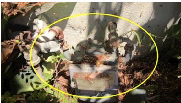
"Rusted" pipe @ gas meter assembly
