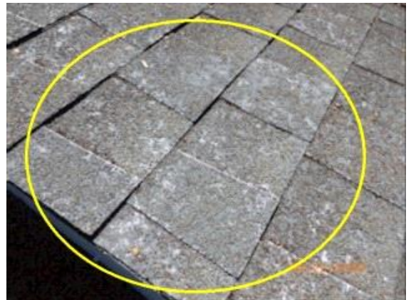
Eroded granular surfaces
