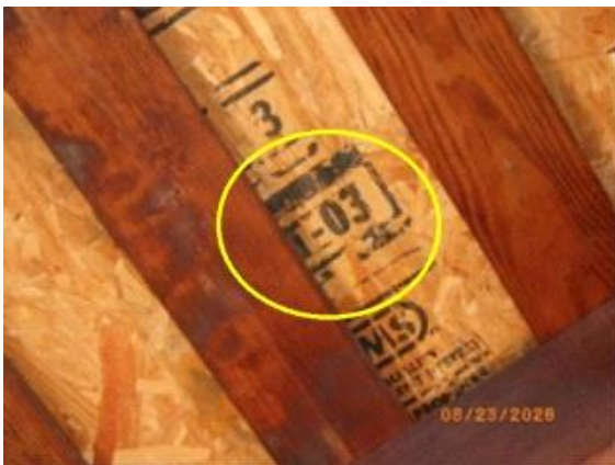
Suspected date stamp observed @ internal roof sheathing
