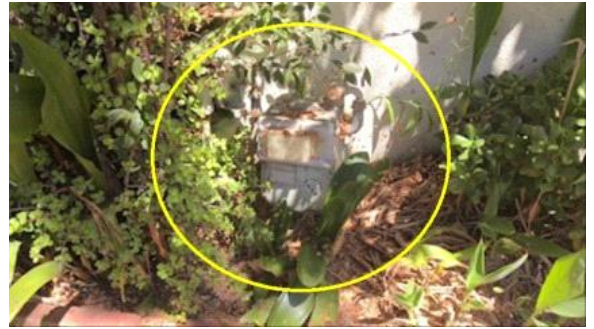
Gas meter intact
