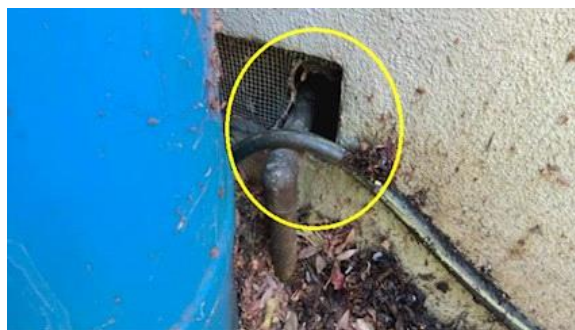
Deteriorated, damaged or misaligned vent screens
