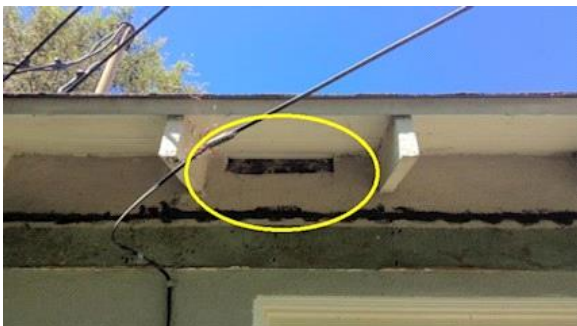
Obstructed soffit vents @ internal attic
