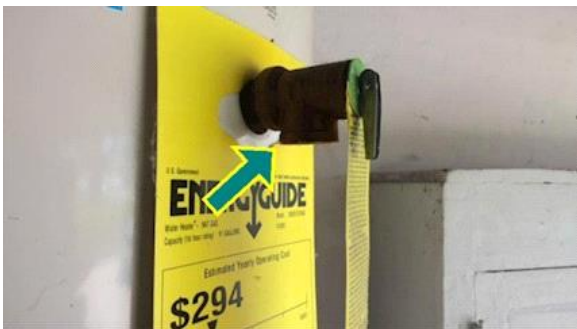
Missing TPRV drain pipe assembly
