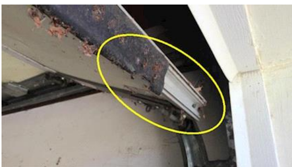
Detached, altered / partially missing weather strip
