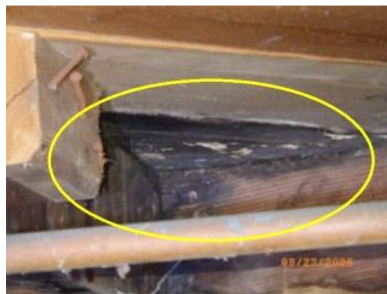
Black-like discoloration observed @ sub flooring
