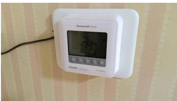
Thermostat(s) intact & observed functional
