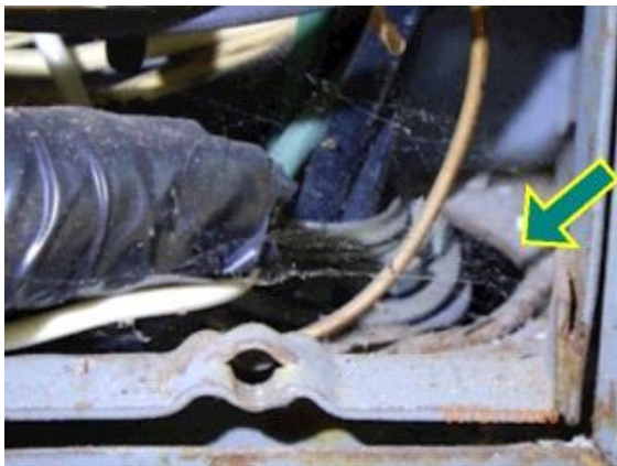
Detached / unsecured internal electrical panel box connector
