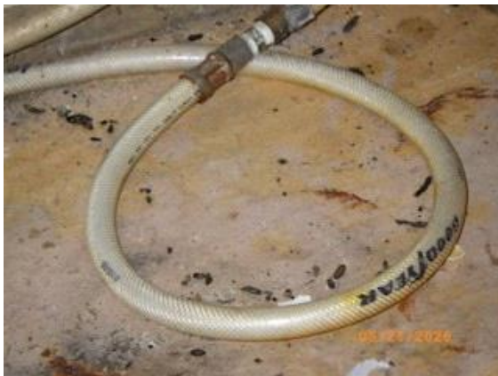
Rodent feces observed below kitchen sink
