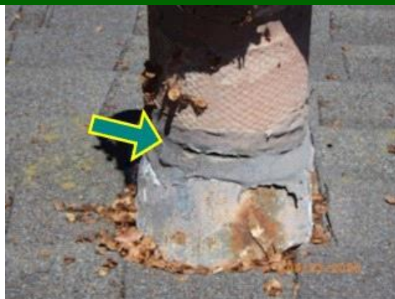
Ex.#1: Cracked / deteriorated mastic sealant
