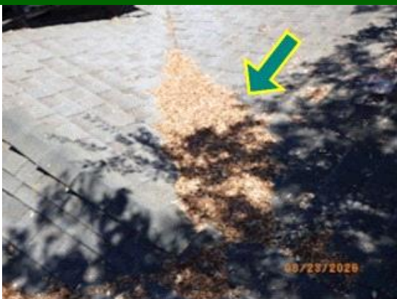
Debris filled valley
