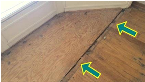
Altered / unfinished flooring surfaces
