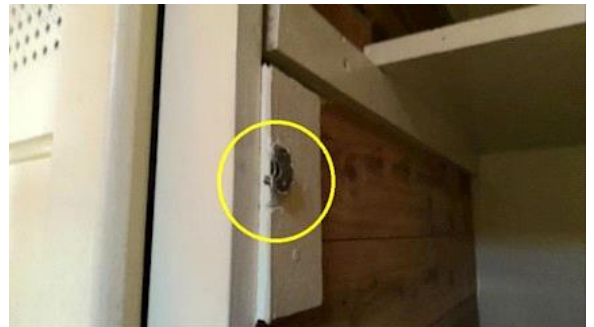
Altered / missing cabinet door latch hardware
