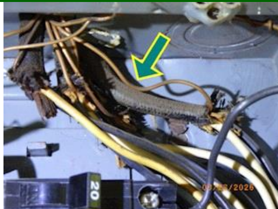
Antiquated conductors / Cloth-wiring observed
