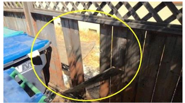
Damaged / missing wood planking
