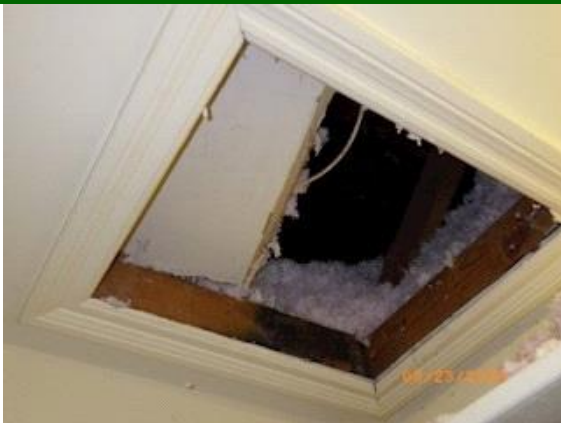
Limited / obstructed interior access
