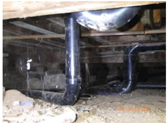
Upgraded plumbing observed @ crawlspace areas
