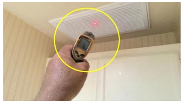
Return temperatures monitored
