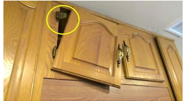
Detached wall cabinet door
