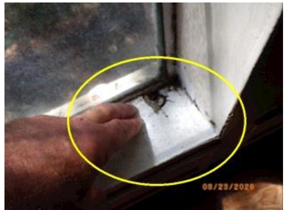
Rotted / decayed window sill surfaces
