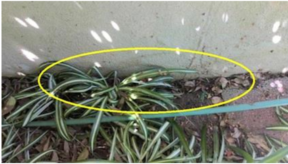
Soil, landscape materials / grading in contact with stucco
