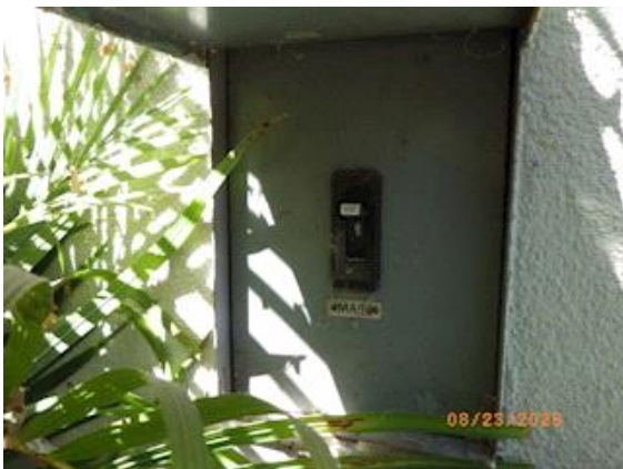
Main disconnect observed secure & intact
