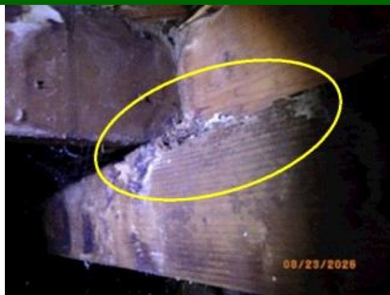
Ex.#1: Wood rot / suspected termite conditions @ framing & support
