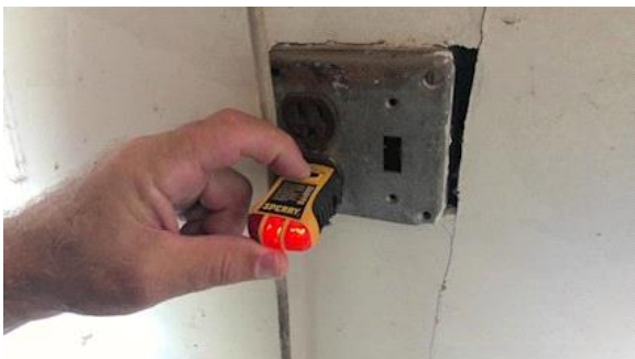
Missing GFCI protection
