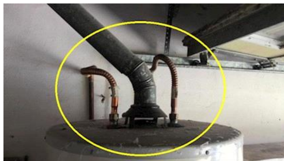
Missing insulated wrap @ supply lines, screws @ exhaust flue & expansion tank
