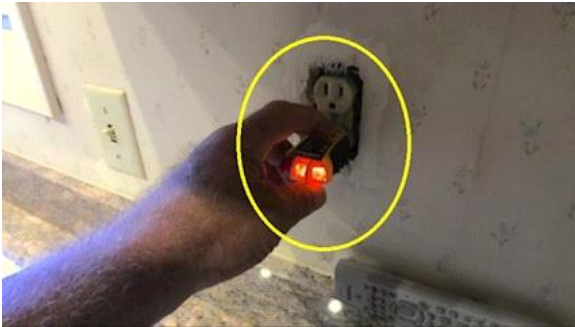
Missing face plate & GFCI protection @ outlet
