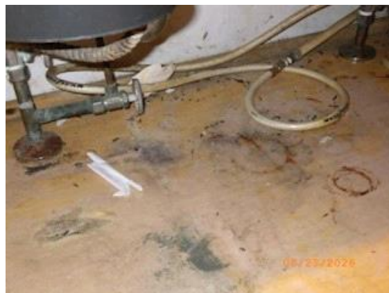
Ex.#2: Stained / deteriorated surfaces below kitchen sink
