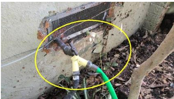
Damaged stucco / Missing vacuum breaker @ hose bib(s)
