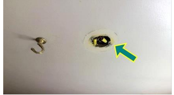
Missing j-box cover / Exposed electrical
