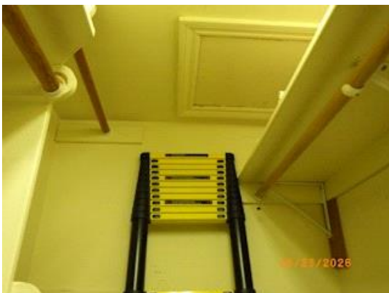
Limited / unsafe attic access
