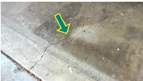
Cracked concrete surface(s)
