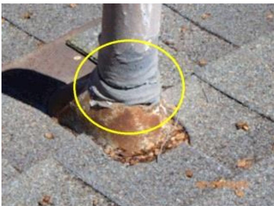
Ex.#2: Cracked / deteriorated mastic sealant
