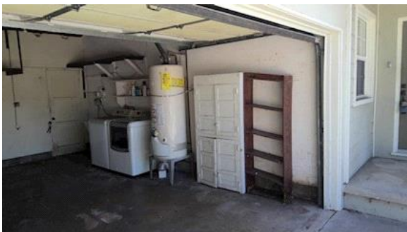
Obstructed / limited interior access & visual inspection
