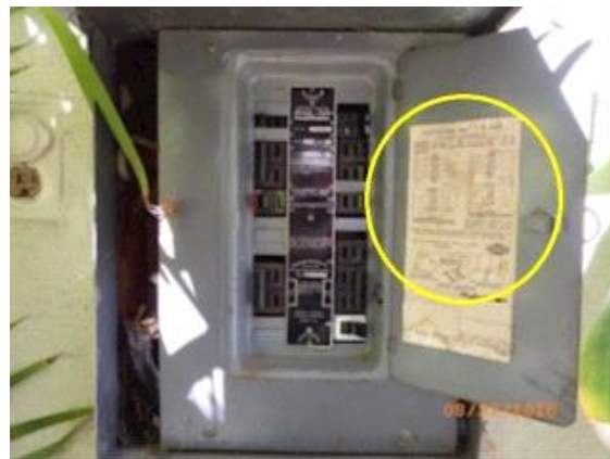
Incomplete, missing or faded circuit breaker labeling
