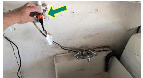
Missing GFCI protection @ electrical outlet
