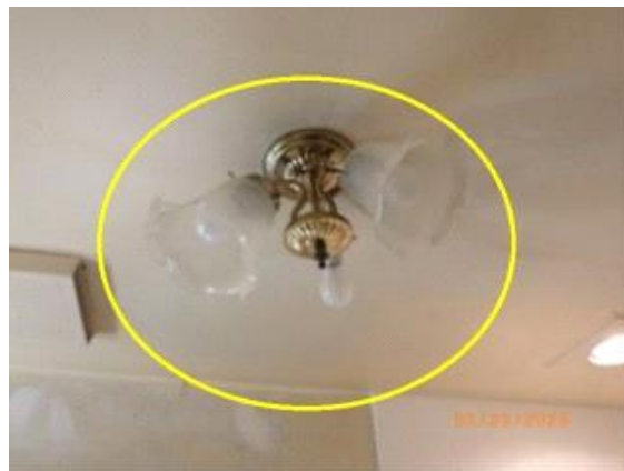
Unconfirmed bathroom ceiling light fixture / Missing protective globe
