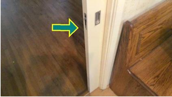
Misaligned / difficult pocket door
