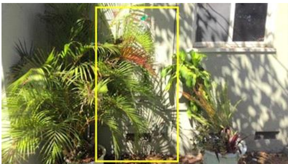
30 x 36 service access obstructed in front of main SE panel box
