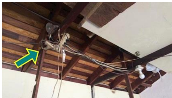
"Mounted" extension cord use
