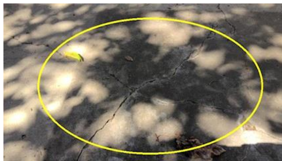
Cracked concrete surfaces
