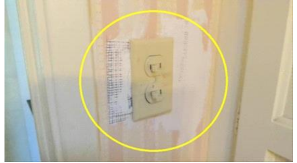
Incomplete wallboard patching
