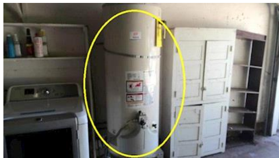
Improper & missing 2nd seismic strapping
