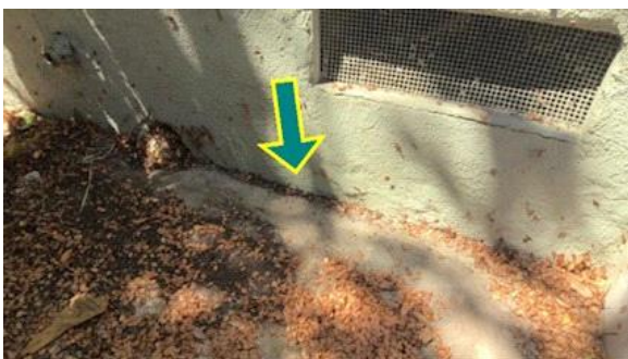
No weep screed / Potential moisture intrusion
