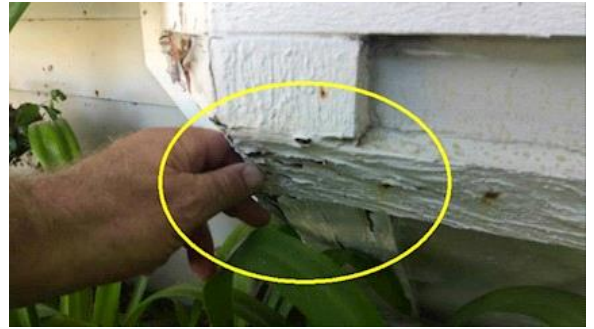
Wood rot, decay and/or suspected termite related conditions
