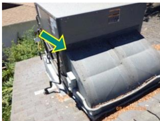
RTU distribution assemblies observed intact
