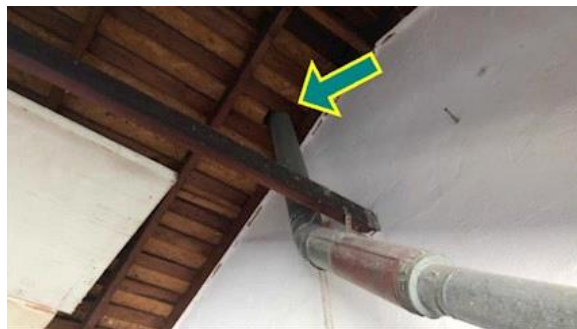
Minimum clearance around exhaust pipe not present
