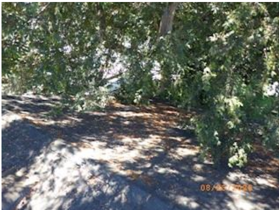
Tree & residual debris in or nearing contact with roof top
