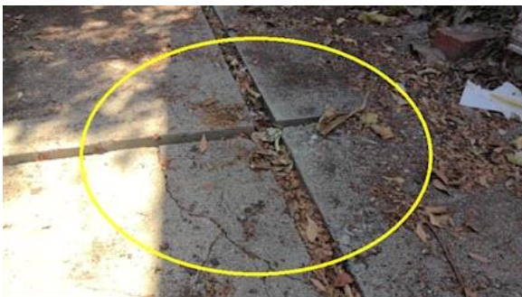
Unlevel surfaces / Recessed expansion joints
