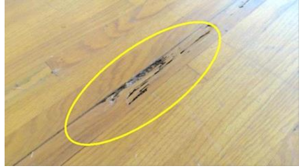
Rotted / decayed wood flooring
