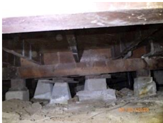
Limited / obstructed interior access & visual inspection
