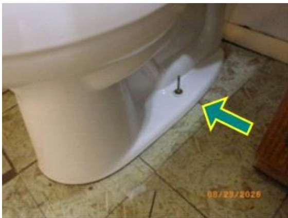
Loose / unsecured toilet mounting
