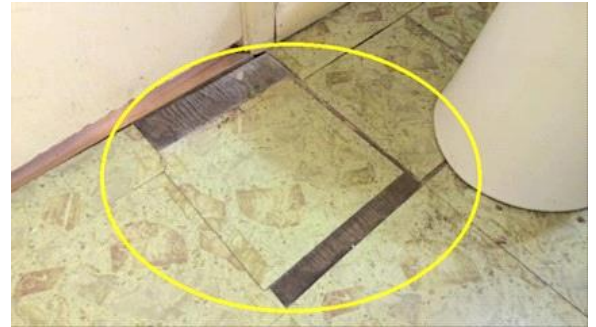
Displaced / loose floor tile
